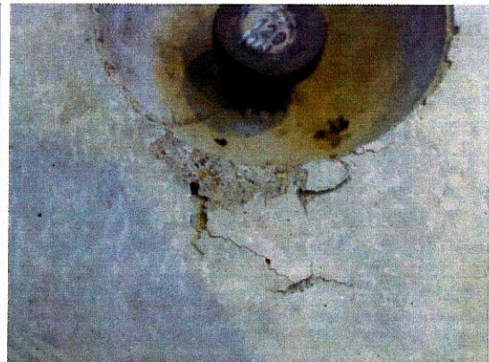
Picture 5 Cracks in concrete block
